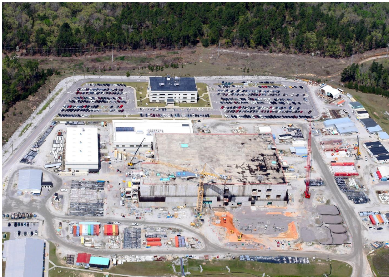
Photo: A view of the south side of the Mixed Oxide Fuel Fabrication Facility (MFFF) under construction at the U.S. DOE's Savannah River Site (SRS) in South Carolina. Note what appear to be 14 Temporary Construction Openings on this facade of the building, open to outside air for many years. Note partially constructed Gabion security wall on outside of facility. More aerial photos available on request. March, 2016, @High Flyer, special to SRS Watch.
