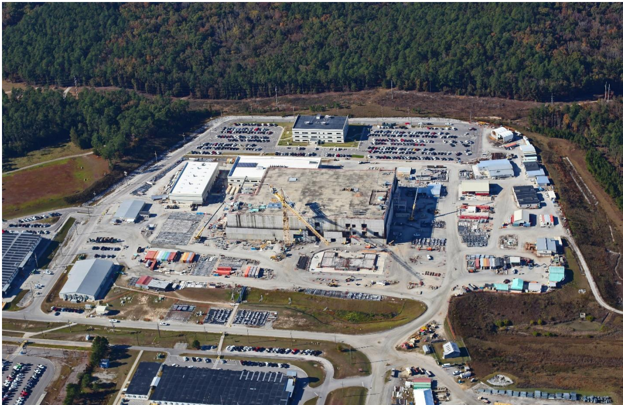
Photo: A view from 2000 feet - the recommended Federal Aviation Administration altitude over DOE facilities - of the Mixed Oxide Fuel Fabrication Facility (MFFF) under construction at the U.S. Department of Energy's Savannah River Site (SRS) in South Carolina, November 10, 2016,
