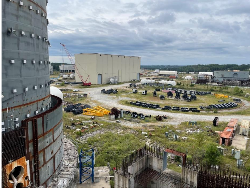
View from the Unit 2 Turbine Building towards the Modular Assembly Building and Unit 3 Containment
