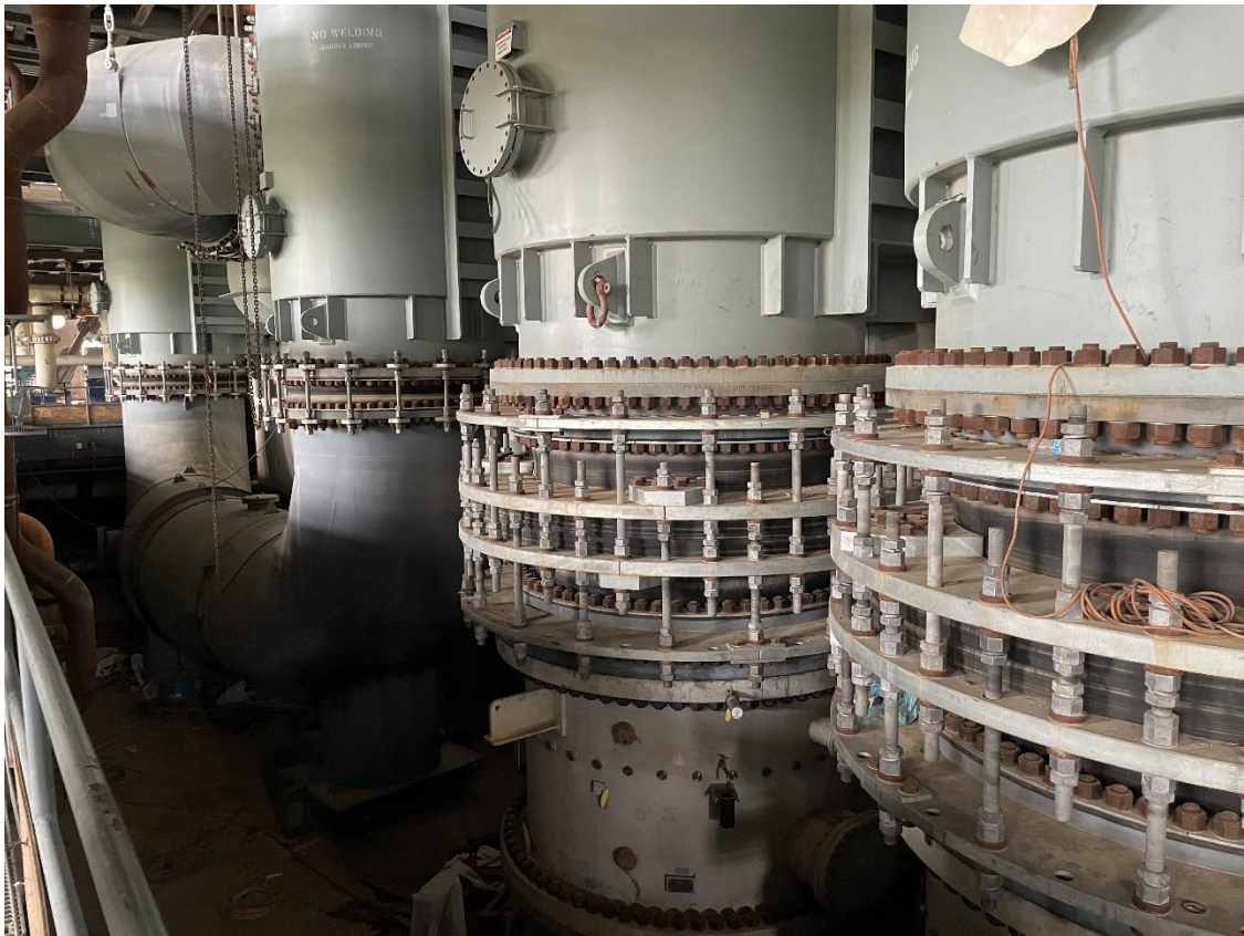
This photo and the following 3 provide examples of installed equipment, piping and structures in the turbine building
