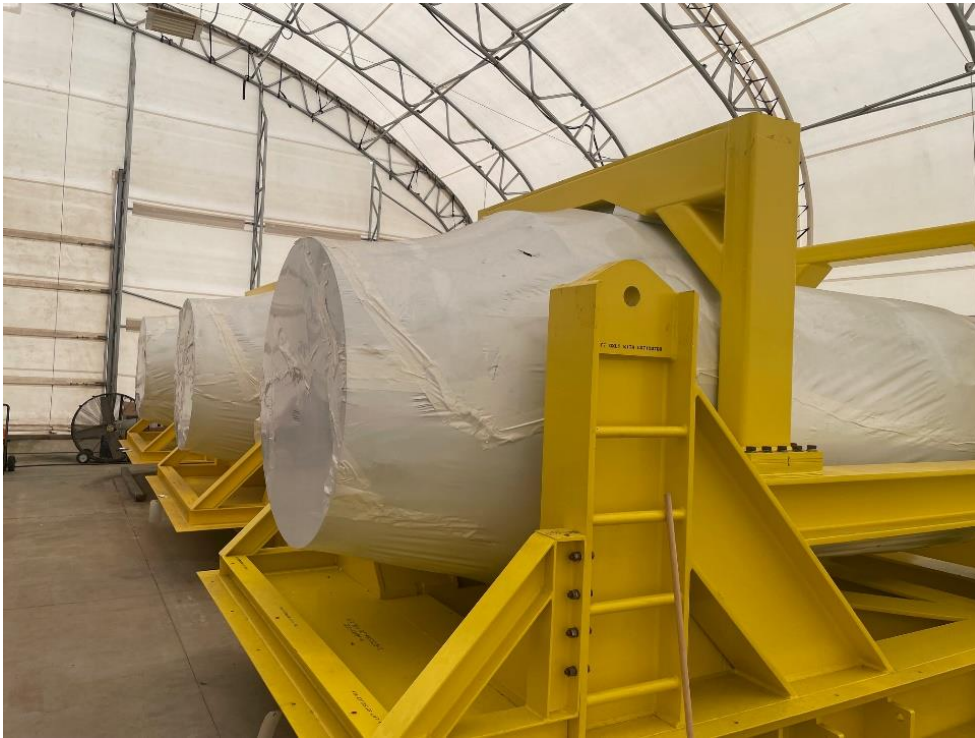
Reactor Coolant Pump storage
