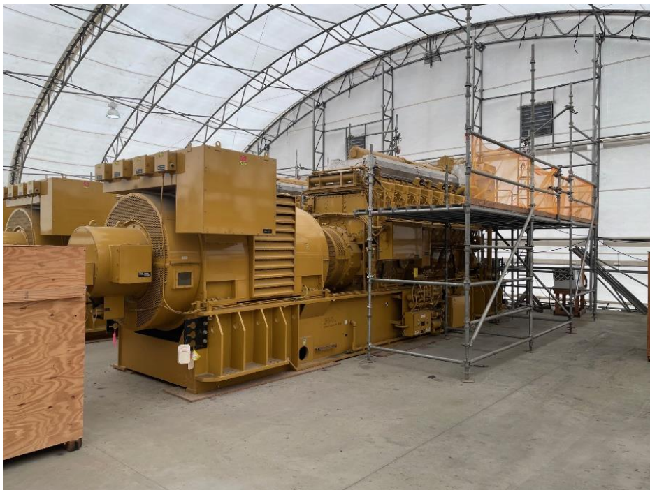
A row of Emergency Power 3500 KW Diesel Generator Packs (4 total) – Regulator Preventive Maintenance is still being performed on the units
